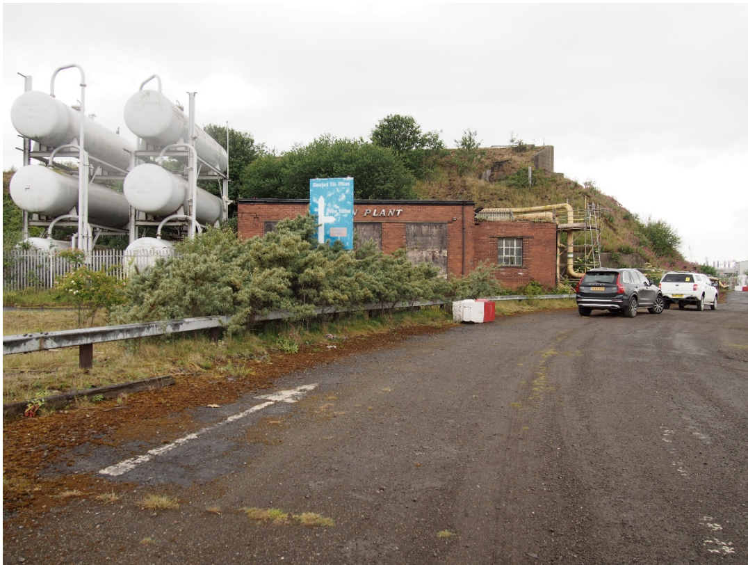
Plate 8: The Oxygen Plant with the embankment of the former railway to the Bessemer Blast Furnaces behind.
